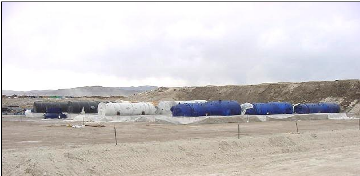
Figure 3-2. Large Component Disposal
